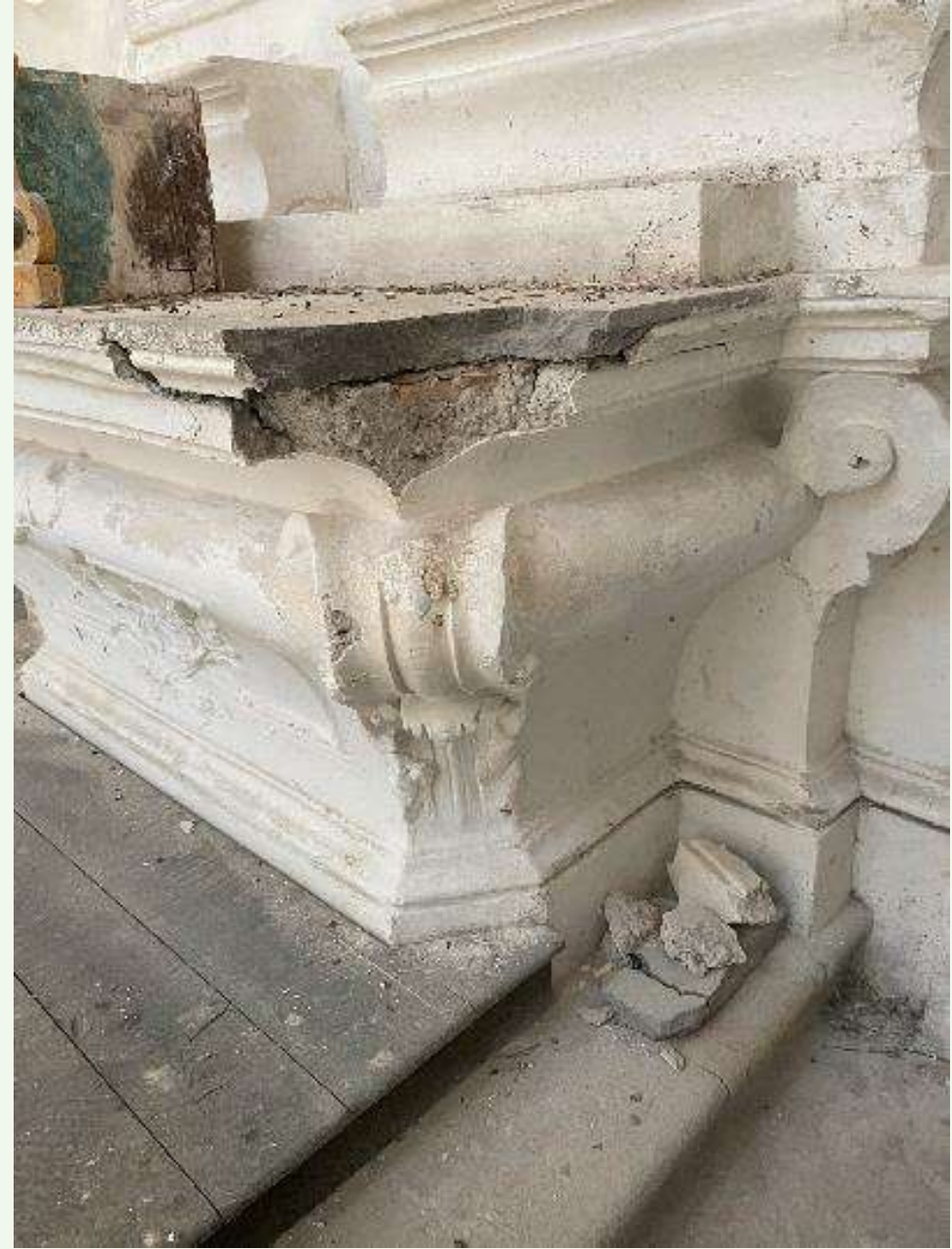
Rainwater infiltrations and cracking of stuccos
