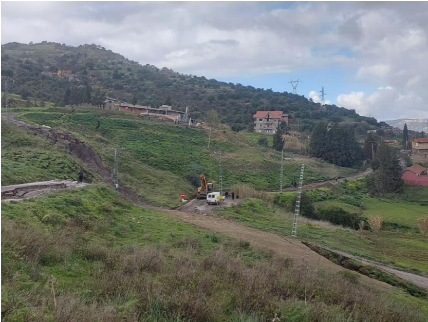
Affected access and field operations after the 25 February 2025 event.
