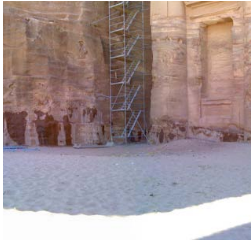
Jordan (Petra) Rising damp, capillarity Seepage (seasonally)
